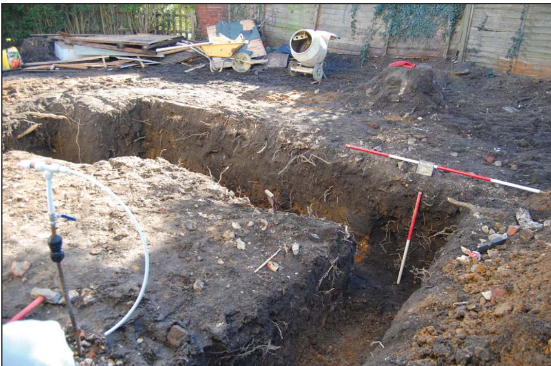
Plate 2. Footing trench for the house extension, looking east, Scales: 2m and 1m.
