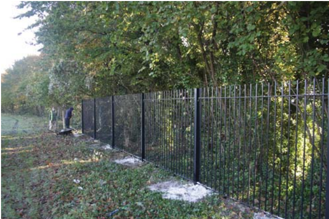
Plate 1. Observation of work in progress.
