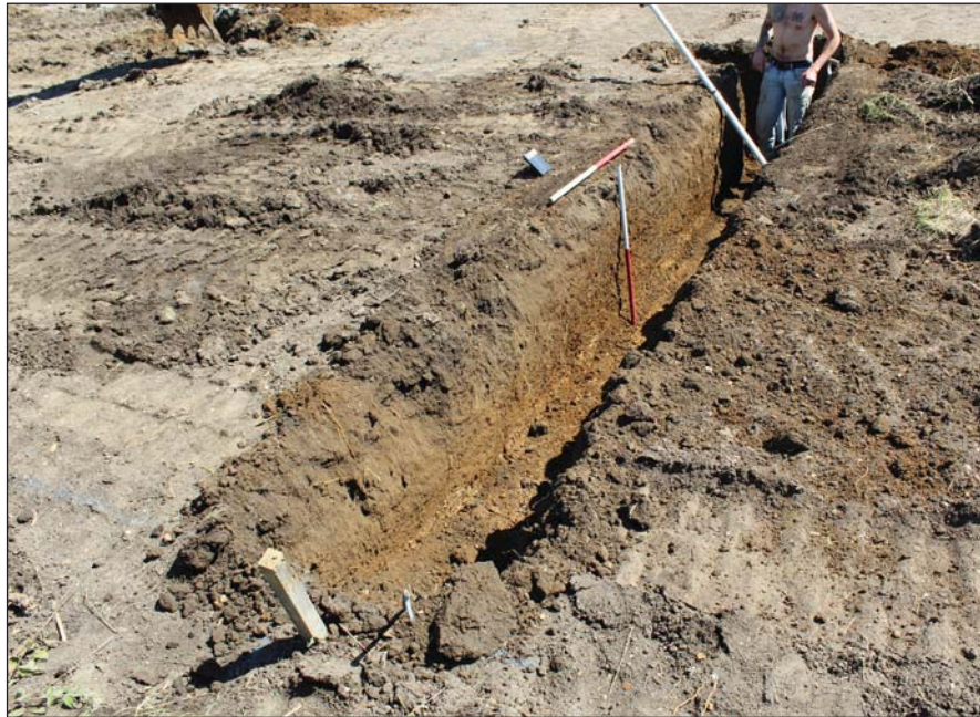
Plate 1. Excavated footing trench on garage, looking north east, Scales: horizontal 1m, vertical 1m.
